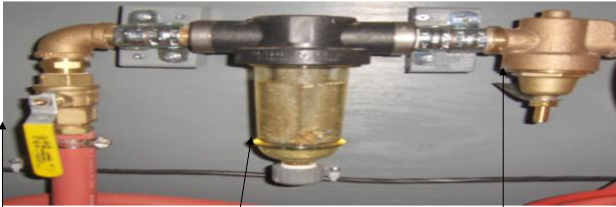
Shut off valve
